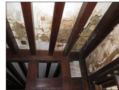
WATER DAMAGED ENTRY HALL CEILING.
