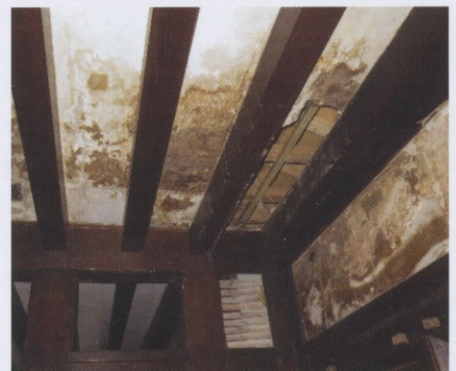
Water damaged main hall ceiling
